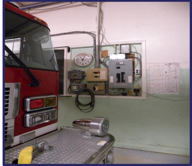
One of Several Electrical Panels
